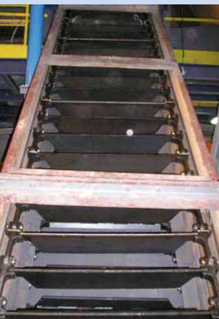
Coal handling conveyor in a power station
